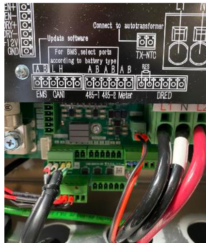
Inverter connections from auto-transformer.
